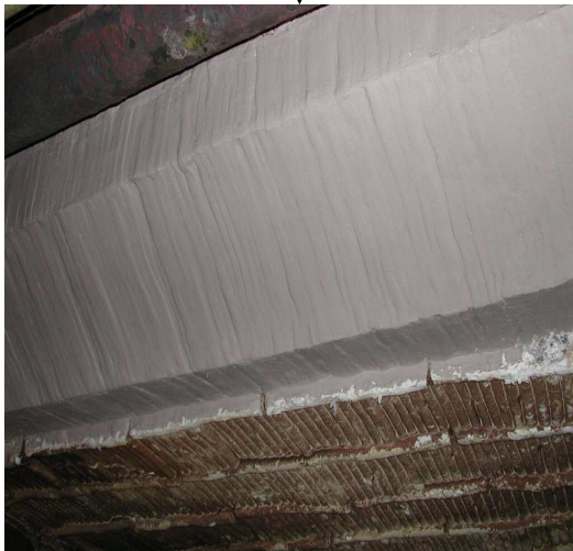
Lintel: Before application
