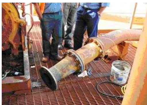
SiSiC Pipe spool being inspected at 2000 hours and going back into service to complete over 8000 hours
